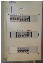
Photo A: Example of House switch board
